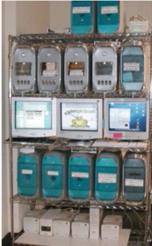
Server Rack At Jett
